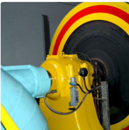
CUNELLA POWER PLANT BERGAMO
